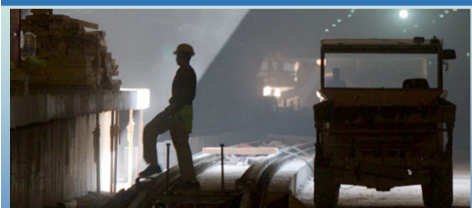
Photo of the month | Work in progress, burying the railway in Palma de Mallorca
